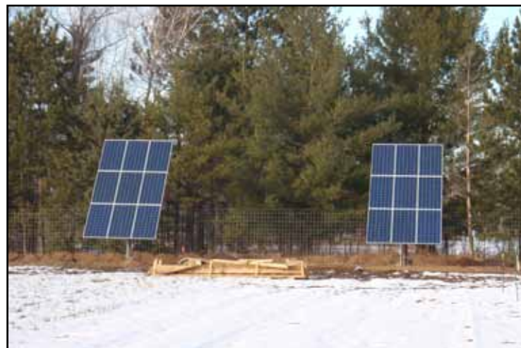
Solar farm at Gitigaaning
