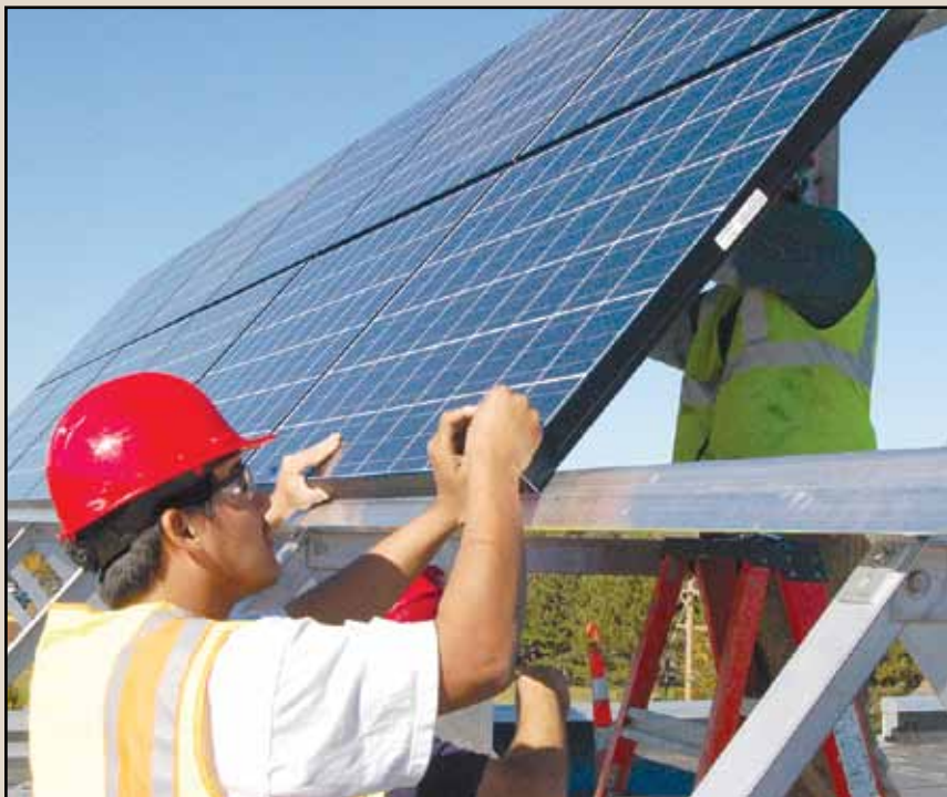
Above: Keith Diver positions one of 57 solar photovoltaic panels during installation on the roof of the Resource Management building.
