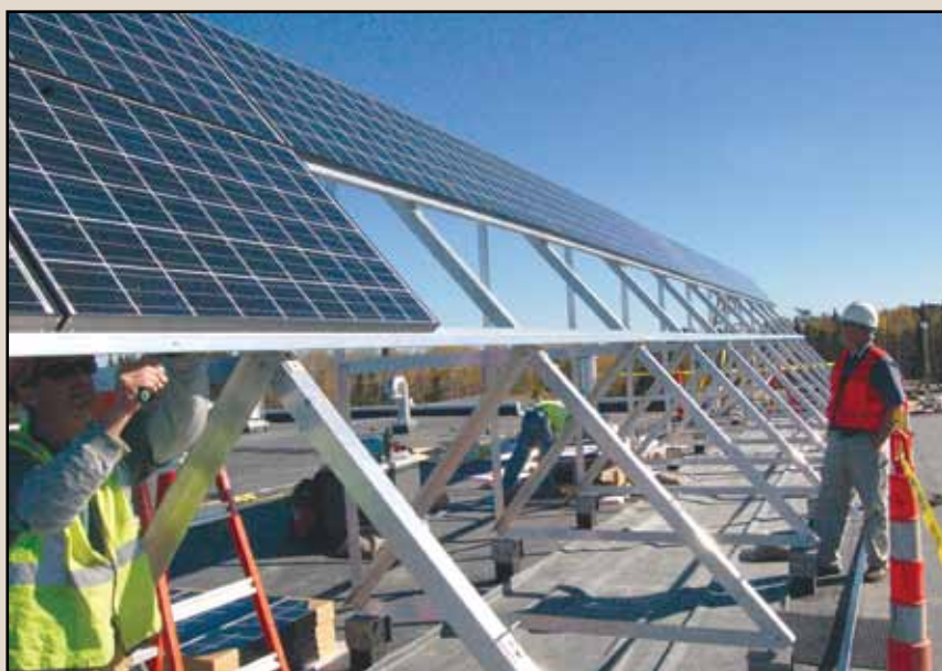
Bottom: Resource Management Environmental specialist Bruno Zagar (right) inspects the progress of the PV panel installation. The 12.25 kilowatt project is the largest of its kind in northern Minnesota, and the second largest solar array project ever installed by Conservation Technologies.
